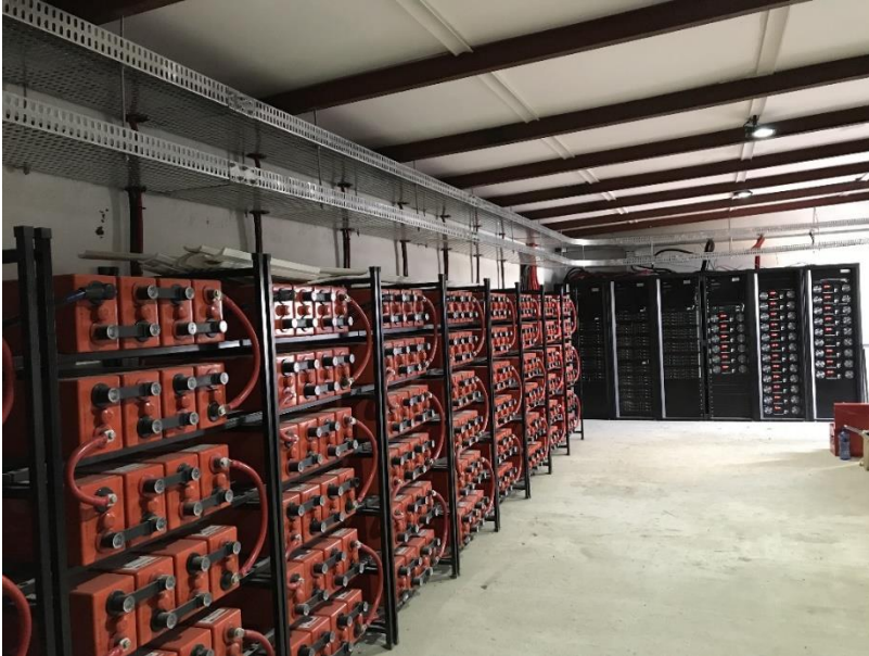
Figure 5: Energy conversion unit and energy storage system at safari lodge in South Africa.
